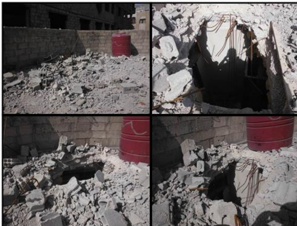
FIGURE A.7.4 CRATER ON THE ROOF OF LOCATION 4
