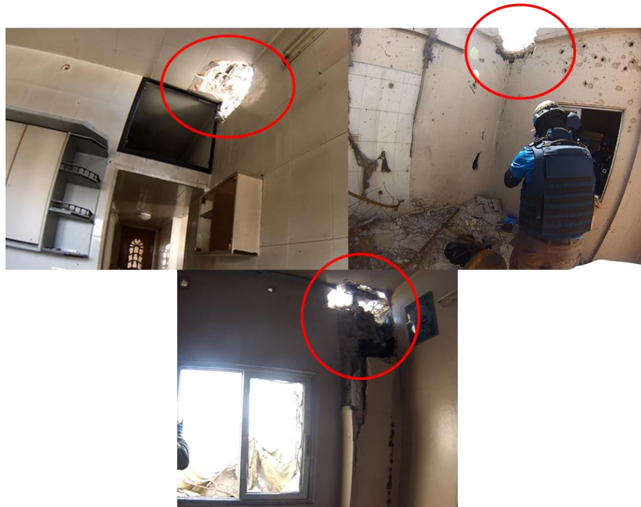
FIGURE A.6.4 DAMAGE ABOVE THE CRATER OBSERVED FROM DIFFERENT ANGLES
